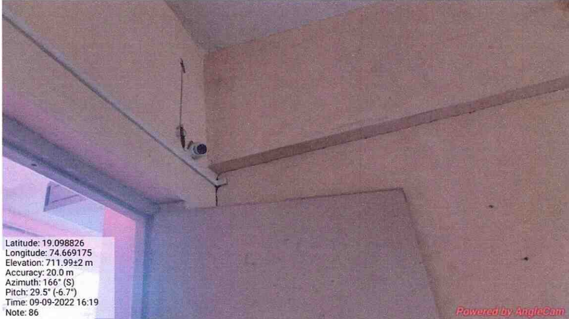
7.1.7.19 CCTV Surveillance inside the classroom
