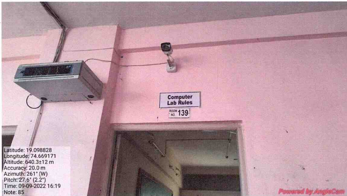
7.1.7.20 CCTV Surveillance outside the Lab
